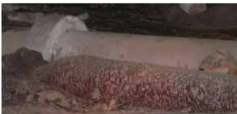
Above: Tree root under Block 2 property, Hastings Street
