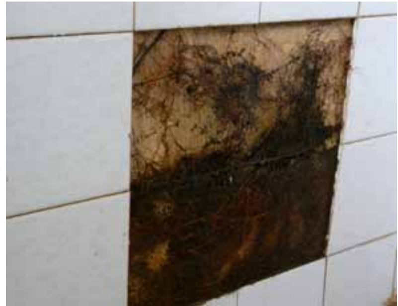
Above: Tree root damage to bathroom, Block 2, Hastings Street
